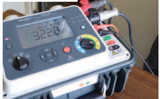
DLRO100H testing rack-mounted, 3-phase circuit breakers
